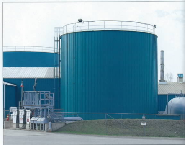
Thermal storage tank
